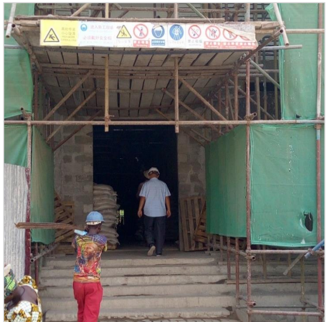
Ongoing construction of JTH Outpatient department with aid from the Chinese government
